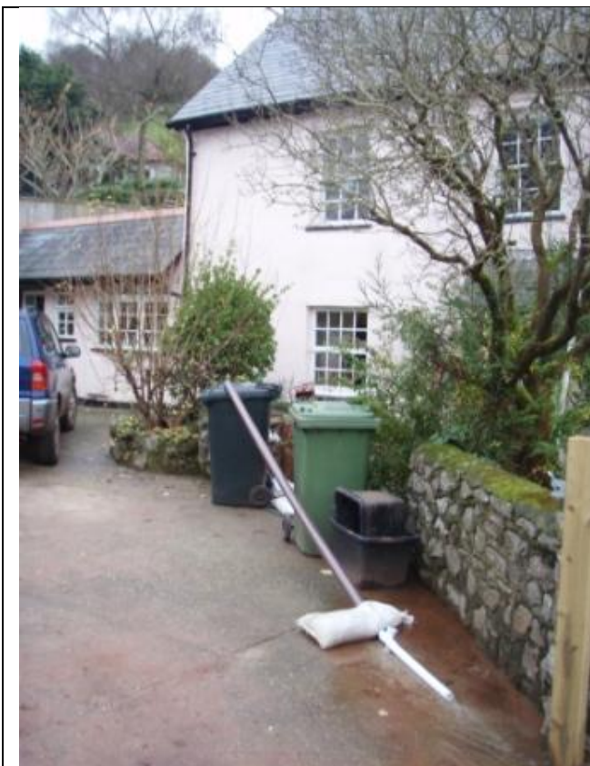
Pumping out well to lower levels at Holly Cottage SX9150870542 looking S
