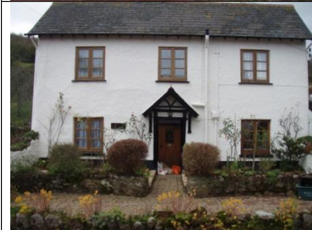
Congdons Farm, some improvised sandbags but there was seepage through the door. SX9162170473 looking W
