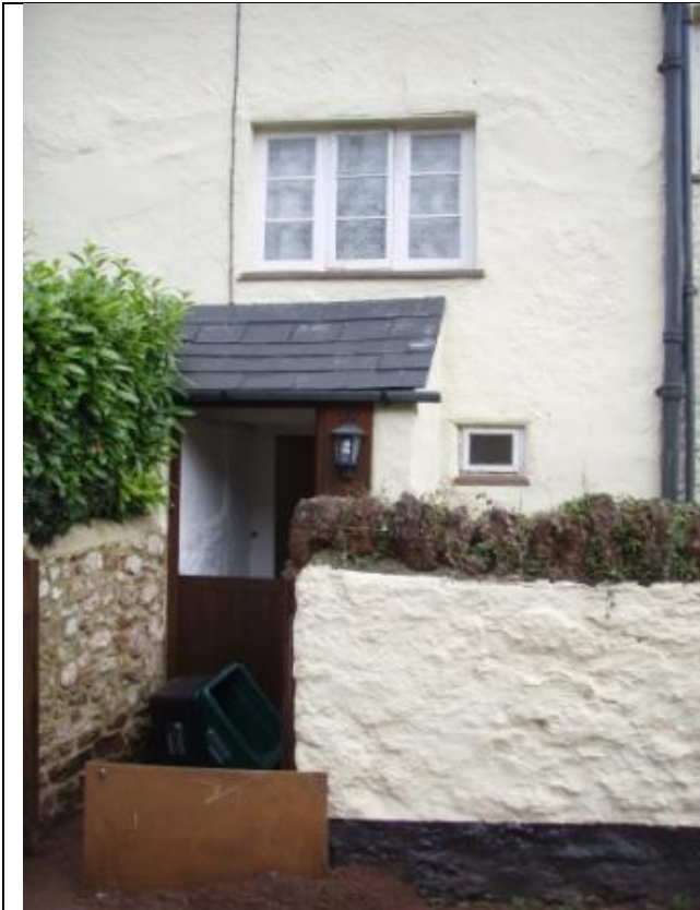
Lower door of Higher Farm which had a small amount of flood water in. SX9166070366 looking E
